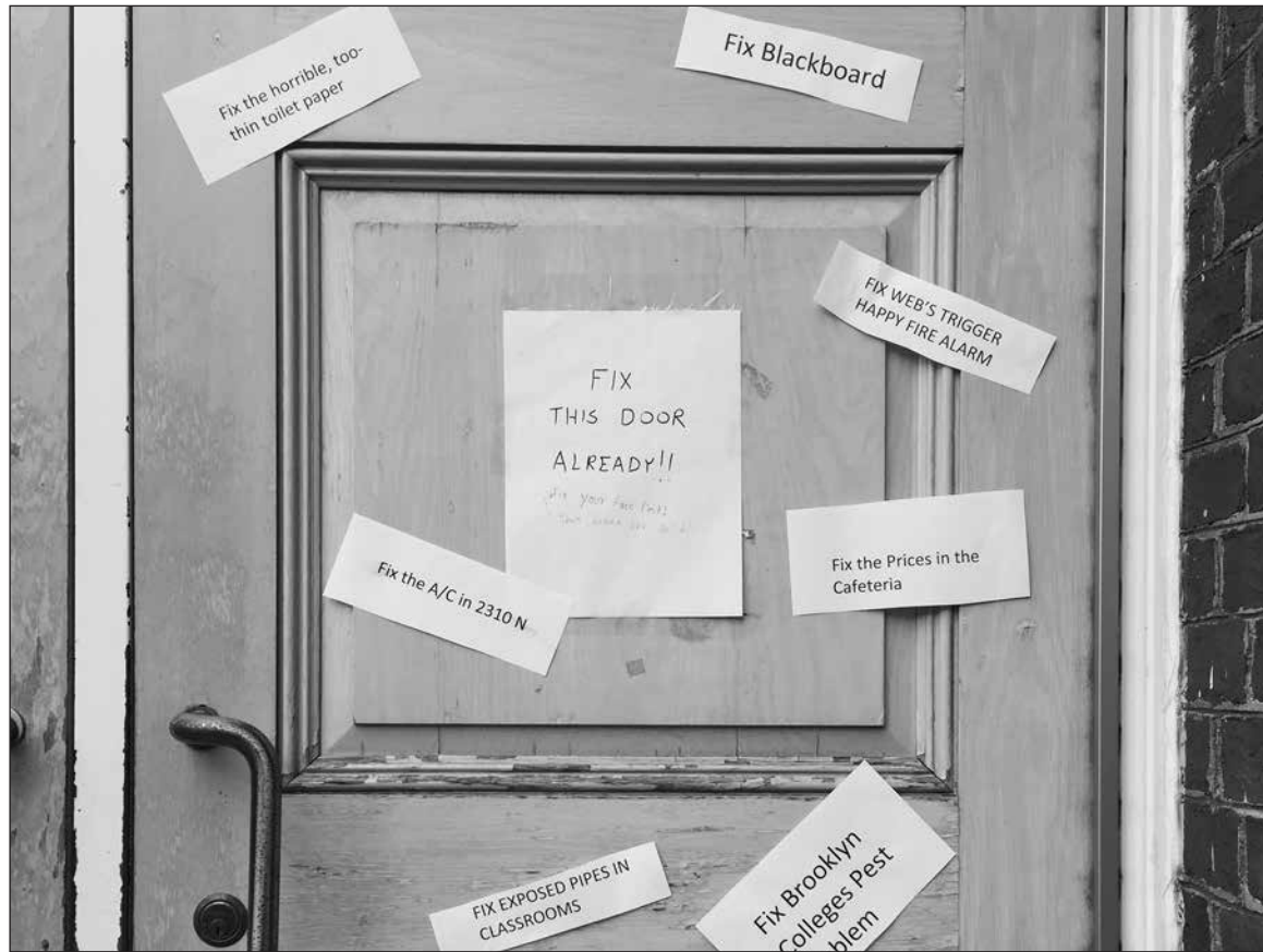
Faculty and students posted pictures of disrepair on social media, including this photo of a broken door to Boylan Hall.
